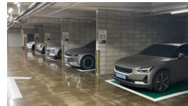
EV Charging Stations at the Pangyo Office
